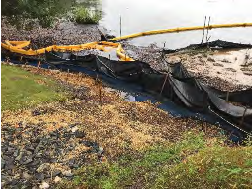
Fig 5: Toe of the slope below the manhole at Gundalow Landing/east side of the bay. Viewing south. (08-29-20).
