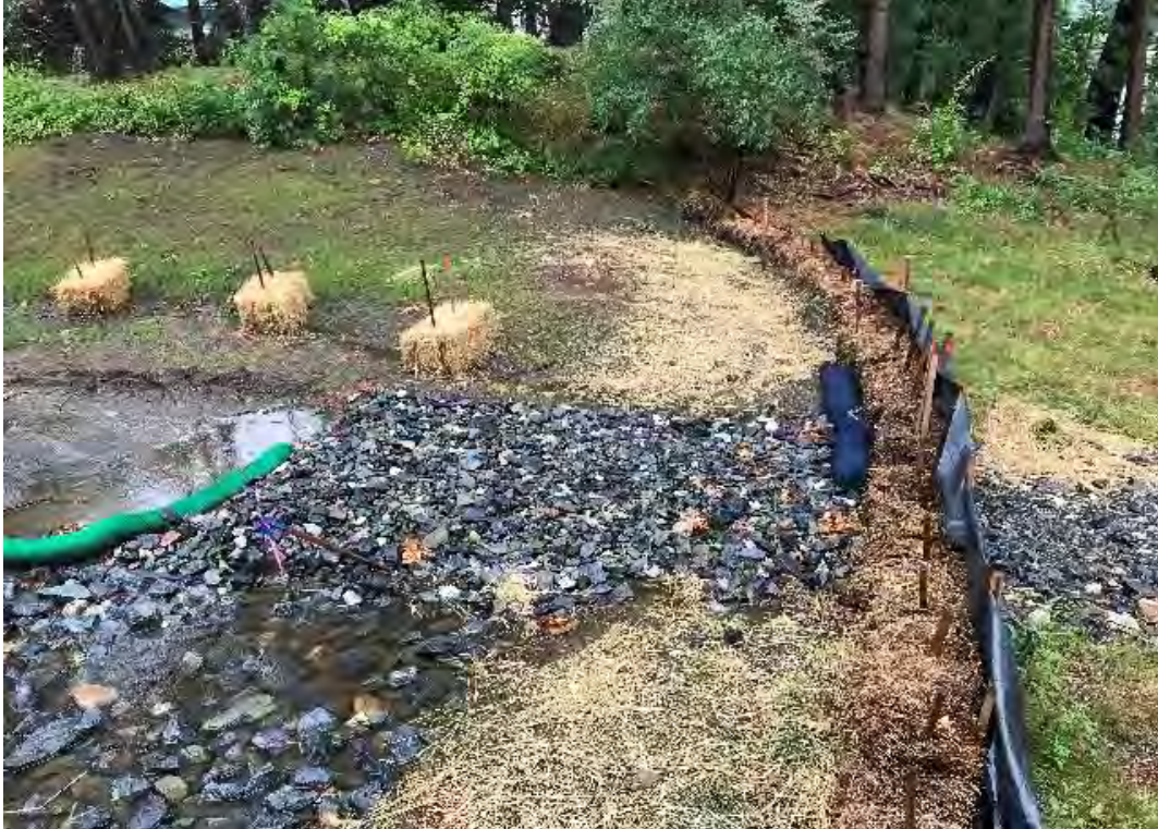
Fig 3: Bottom of the slope above the manhole at Gundalow Landing/east side of the bay. Viewing south. (08-29-20).
