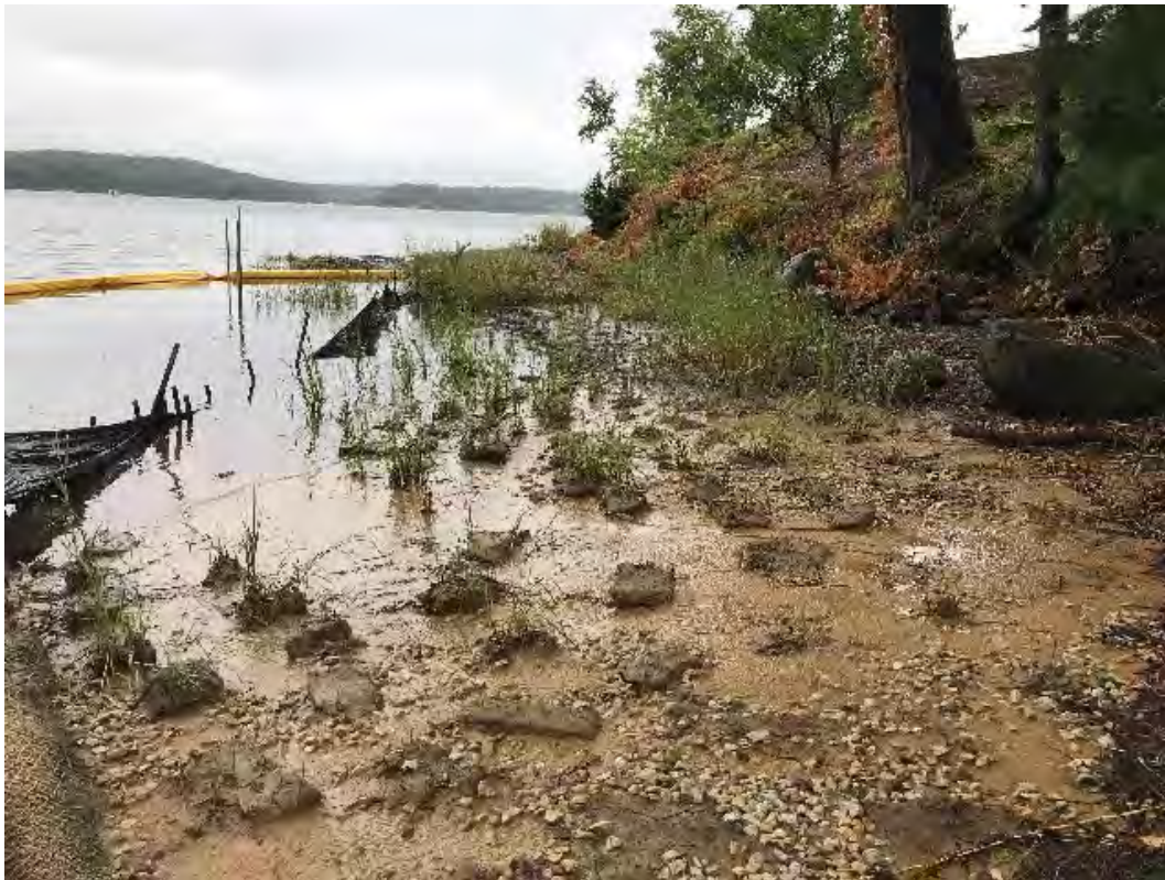
Fig 6: Salt marsh restoration at Gundalow Landing/east side of the bay. Viewing northwest. (08-29-20).
