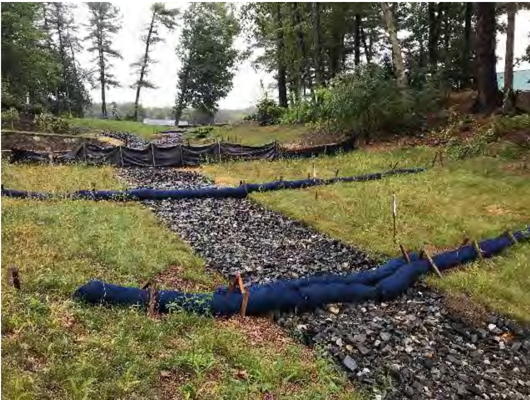
Fig 4: Slope below the manhole at Gundalow Landing/east side of the bay. Viewing northeast. (08-29-20).
