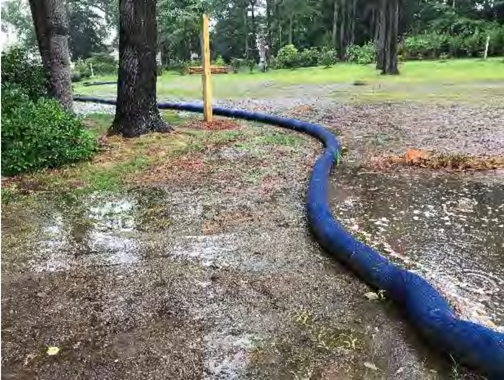
Fig 1: Silt sock on southern side of Beswick property at Gundalow Landing/east side of the Bay functioning as intended. Viewing northwest. (08-29-20).
