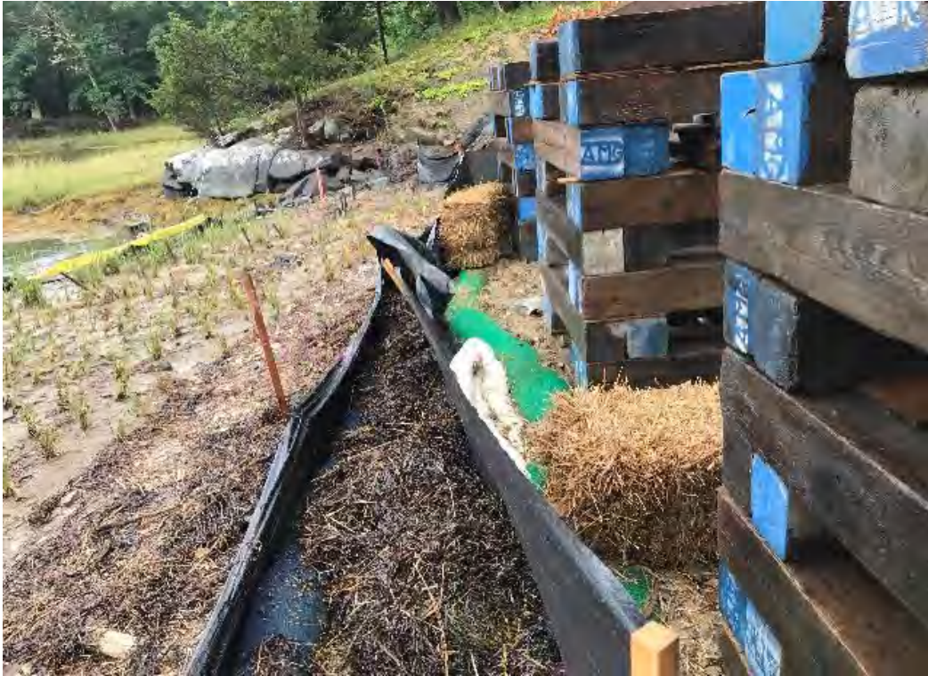
Fig 9: BMPs below the new cable house foundation at the Eversource property/west side of the bay are functioning. Viewing south. (08-29-20).
