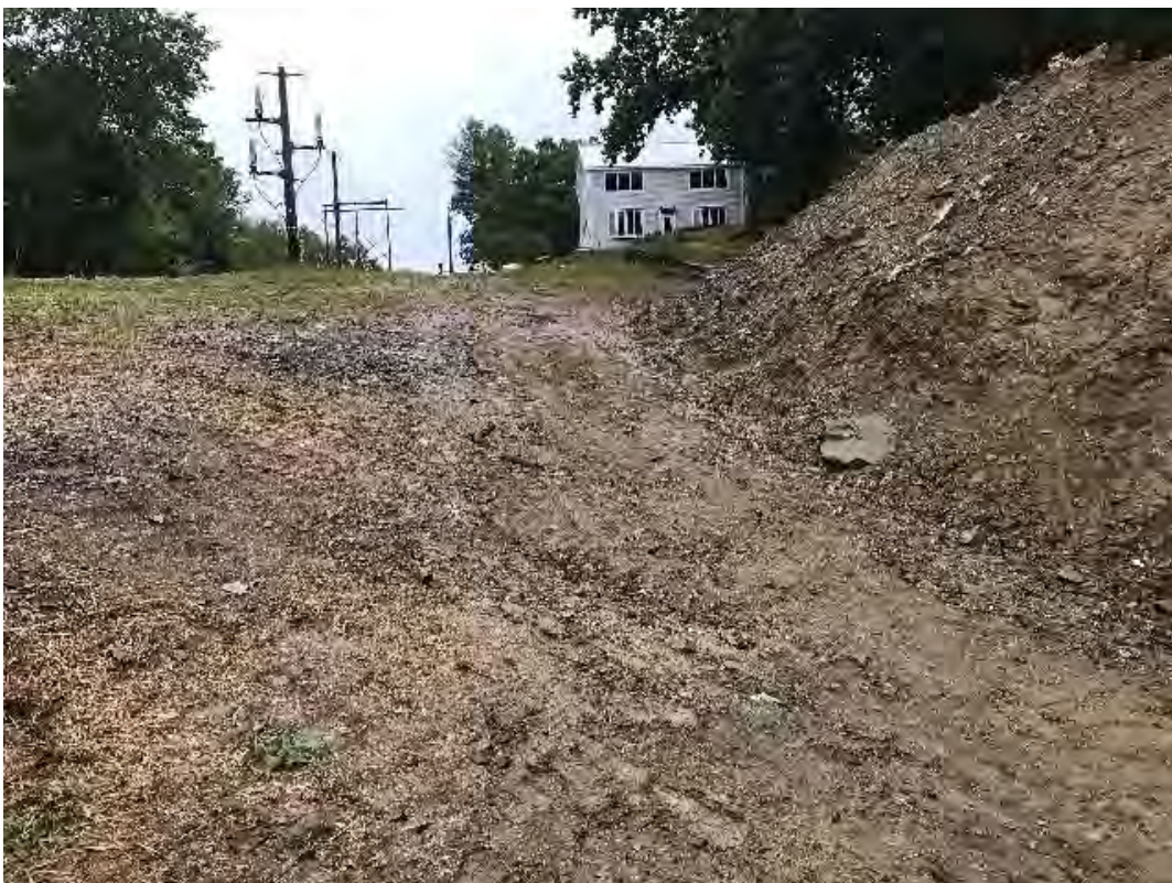
Fig 8: The slope above the new cable house location at the Eversource property/west side of the bay is stable. Viewing west. (08-29-20).
